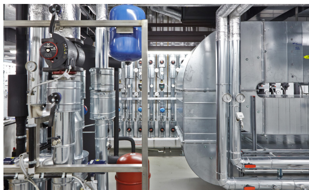
Technical plant room
