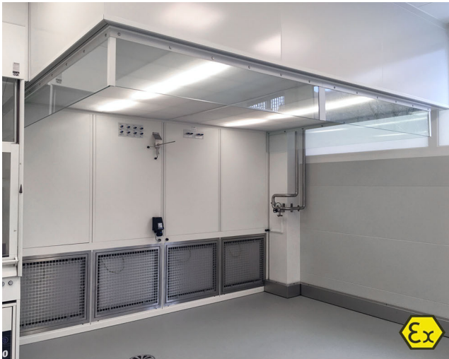
ATEX-Anlage / ATEX system
