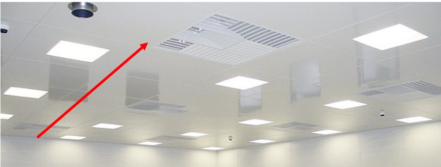
The Plenum Integrated Filter Fan Unit (PIFF) installed in a cleanroom ceiling
